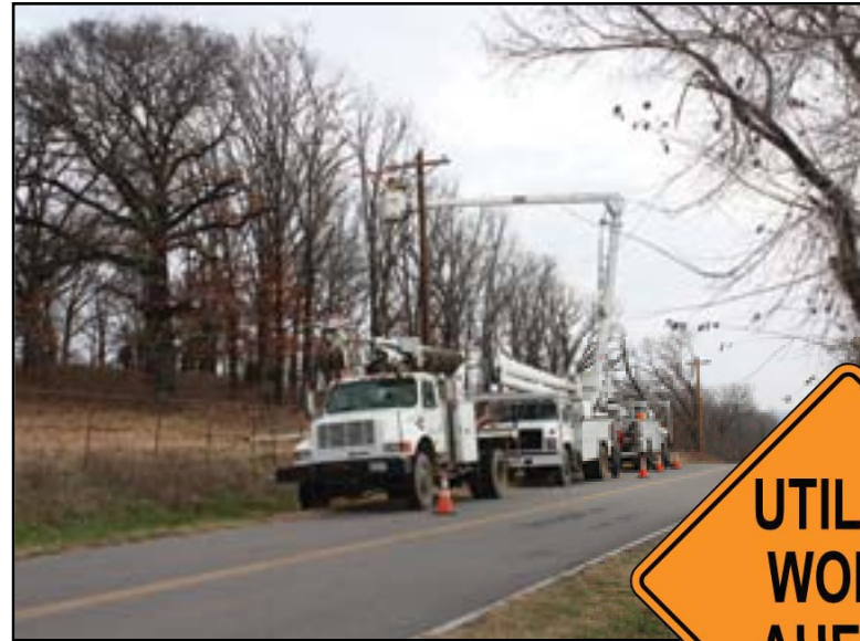
Tech Line Electrical Contractors working off highway 64B east of Sallisaw. Photo by: Larry Mattes
